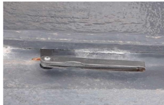
Figure 11. Continuation of the crack at the port-side (Br) bow corner of the Rayo's mast, with a 0.9 mm feeler gauge inserted
